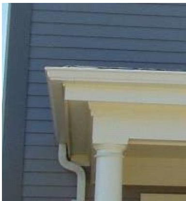
32.2 Ogee gutters should return with the eave or entablature and die into the face of the house.
